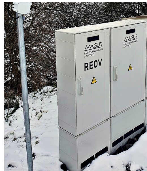
REOV control cabinet and sensor mast beside the track
