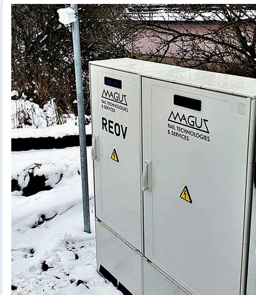
REOV control cabinets – side view with sensor mast
