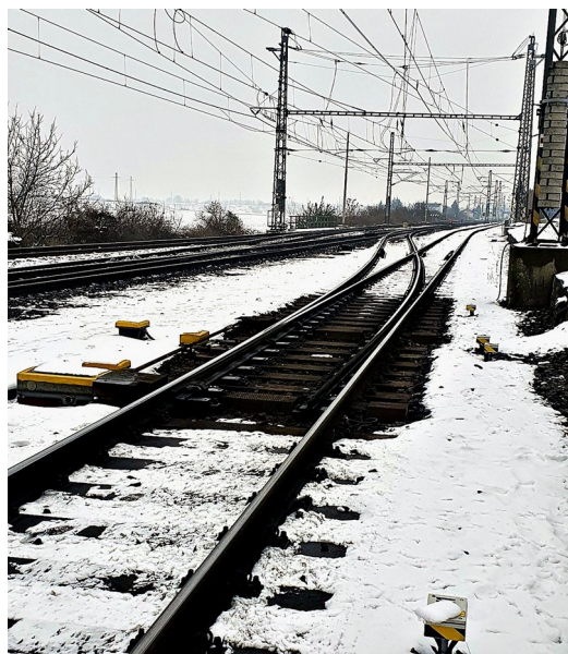
Turnout with MAGUS EOv heating in winter conditions
